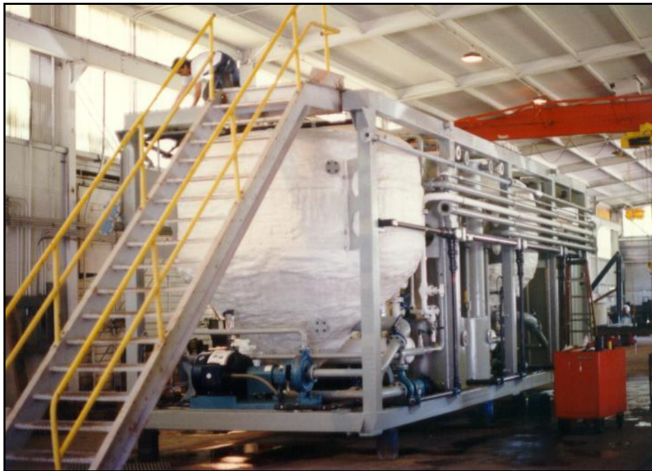
Photo #8. One of modules installed it the railroad car tanks washing shop.
