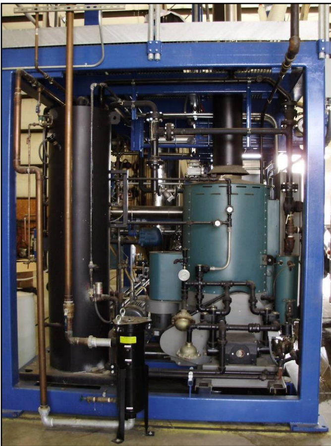
Photo #6. Water cleaning system.
