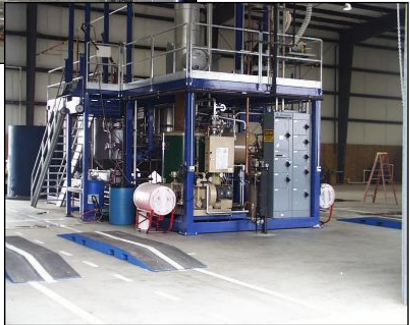
Photo #1. General view of automated washing system for two tank trucks (two views).
