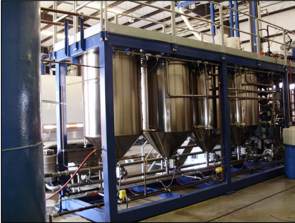
Photo #7. System main frame.
