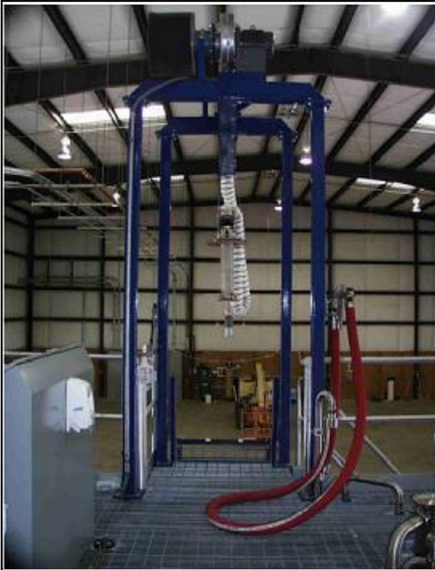
Photo #3. Adjustable gangway platform with manway adapter.
