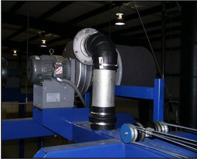
Photo #9. Induced draft fan.
