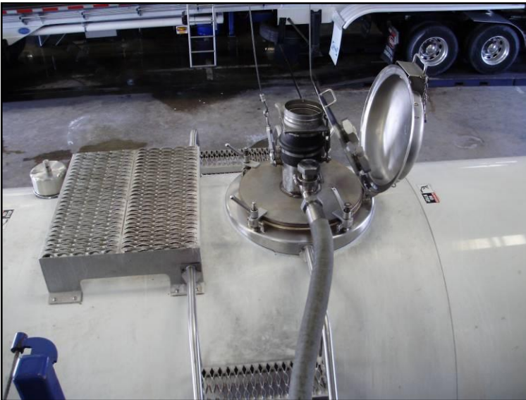
Photo #4. Manway adapter installed on the top manway of the tanker truck.
