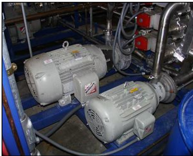
Photo #8. Pumps mounted on the frame.
