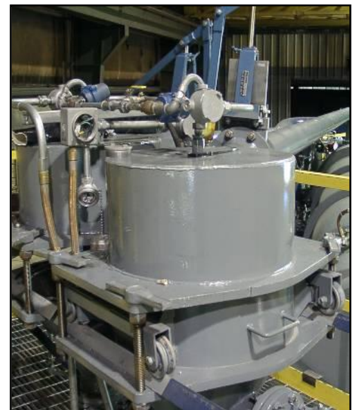
Pic. 6. Mist eliminators.
