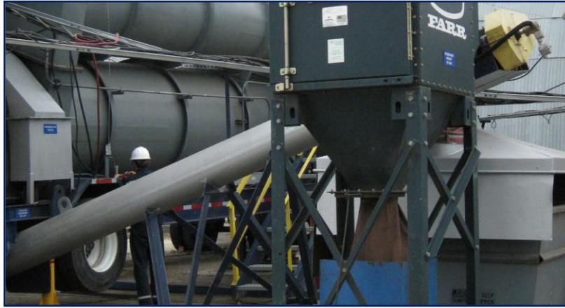
Pic. 7. Unloading and cooling system.
