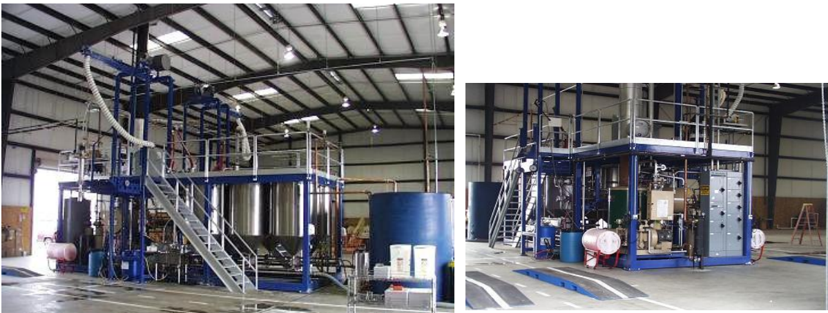
Photos 1a and 1b. General views of automated washing system for two tank trailers
